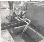
FLOW METER AT INLET TO MAINTAIN THE FLOW OF SEWAGE
